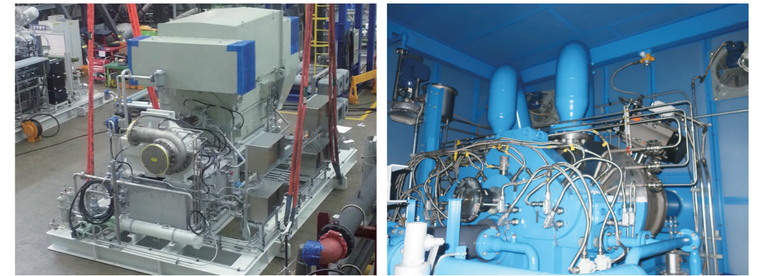
MENA Power Plant FGC
