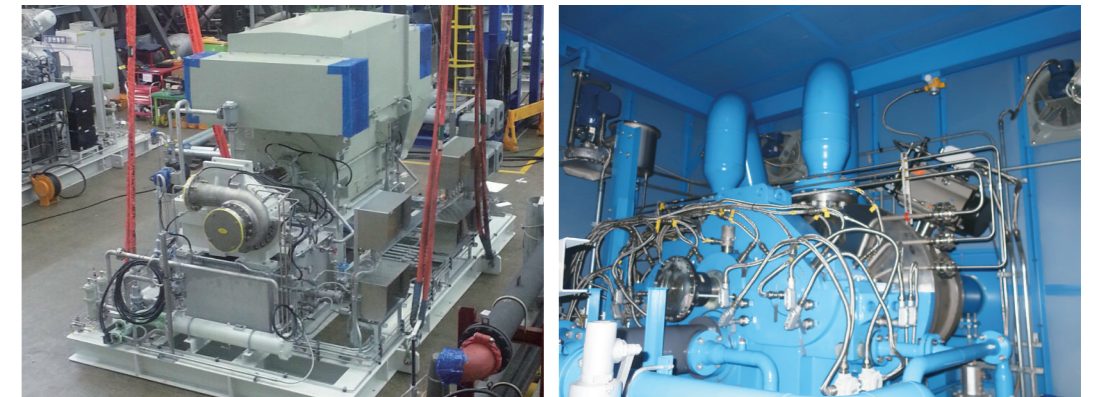
MENA Power Plant FGC
